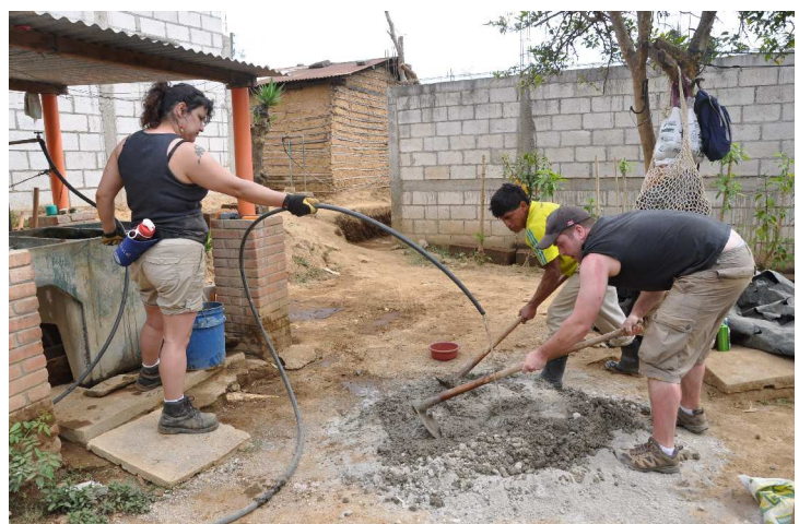
Seemingly endless amounts of mud for blocks and cement for foundations needed to be mixed
